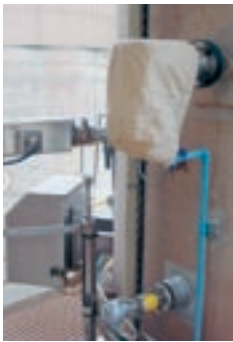
Continuous emission monitoring equipment in place
