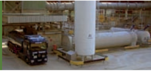
Storage and dosing for waste
