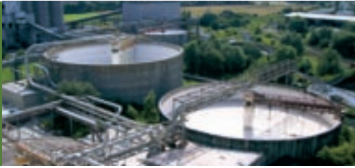
Slurry storage tanks
